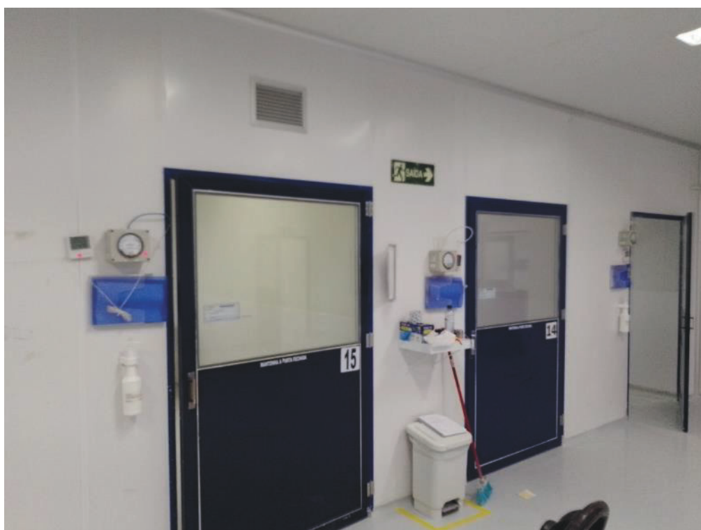
ITENS 1,514 / 1,515 / 1,516 / 1,517 / 1,518 / 1,519 / 1,520 / 1,521 / 1,522 / 1,523 / 1,524 / 1,525 / 1.526 - MEDIDORES DE TEMPERATURA MANOMETROS MAGNEHELIC
