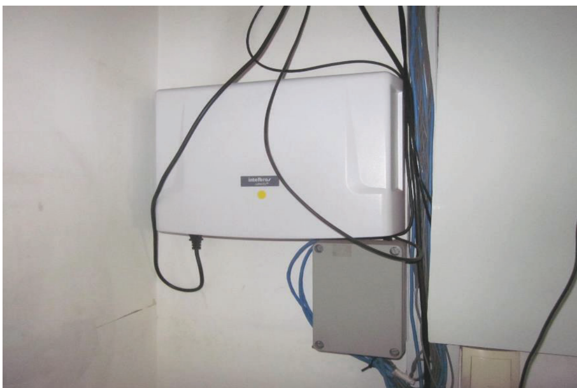
ITEM 1,790 - CENTRAL PABX INTELBRÁS IMPACTA 8I
