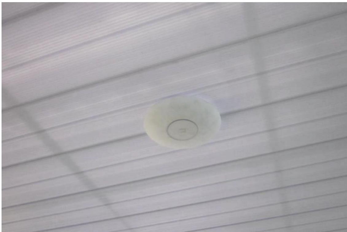
ITEM 1,740 - ACCESS POINT UBITQUI UNIFI1.300 MPBS
