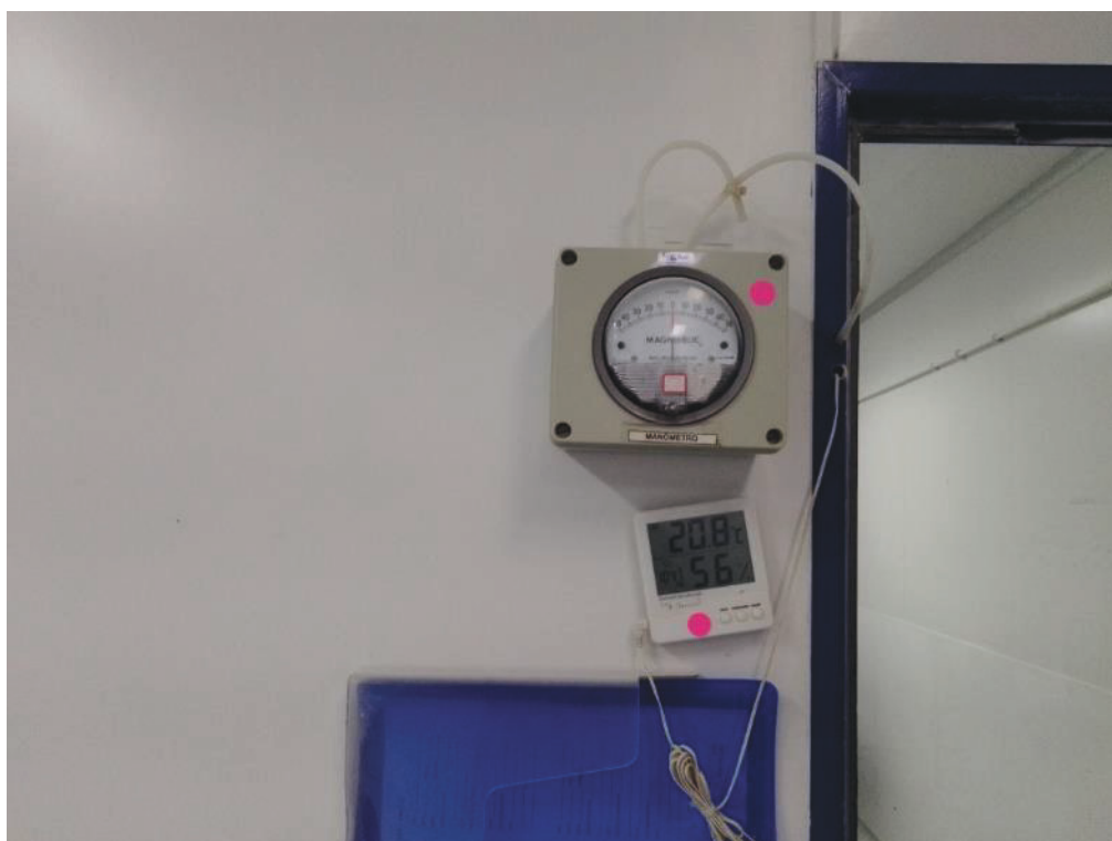
ITENS 1,514 / 1,515 / 1,516 / 1,517 / 1,518 / 1,519 / 1,520 / 1,521 / 1,522 / 1,523 / 1,524 / 1,525 / 1.526 - MEDIDORES DE TEMPERATURA MANOMETROS MAGNEHELIC
